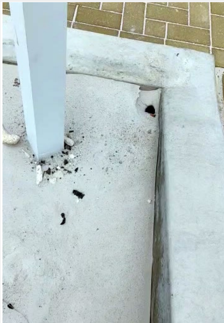
Figure 7. Sand can be seen accumulating along the retention wall.
